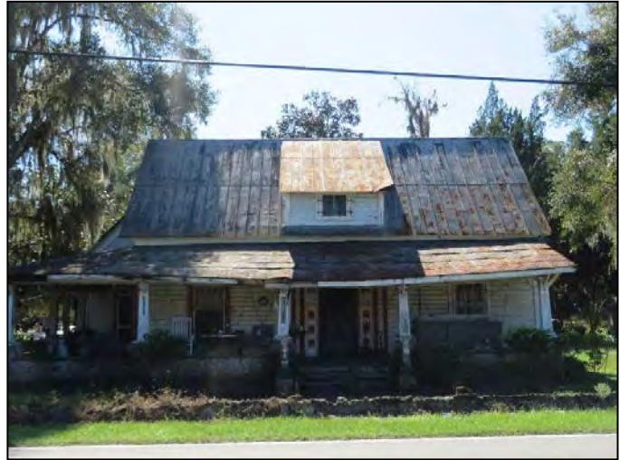
FIGURE 41 | Overview of the Warm Springs Avenue Scatter (8SM00934) site, view south toward 8SM00853.
