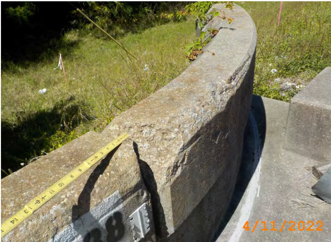
Photo 4: Element 8475: Spall at northeast wingwall barrier at Abutment 6.
