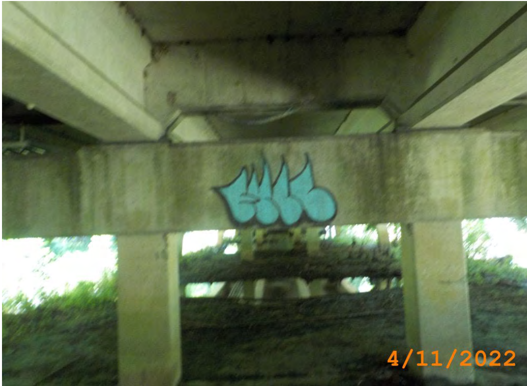
Photo 13: Inspection Notes: Graffiti on Bent 4 cap.
