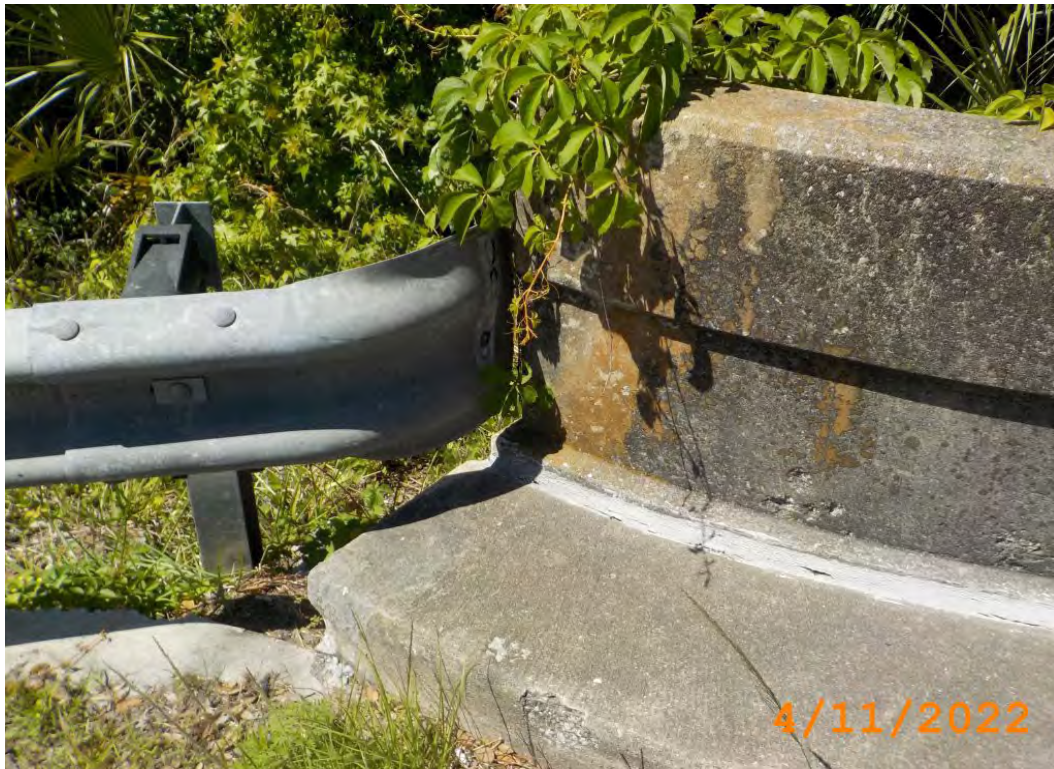
Photo 12: Inspection Notes: Northwest guardrail not attached to structure.
