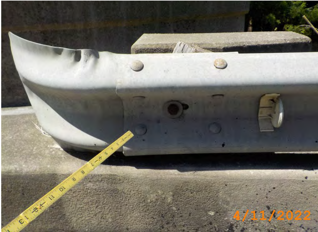
Photo 11: Inspection Notes: Northeast guardrail attached to structure with one bolt.
