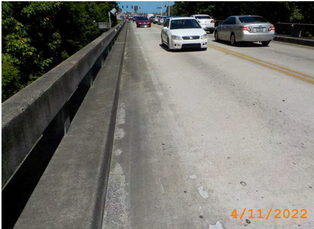
Photo 14: Inspection Notes: Heavily faded and chipped roadway striping.
