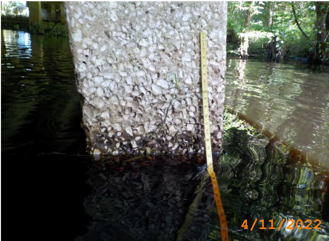
Photo 6: Element 226: Scale damage on Bent 2 pile.
