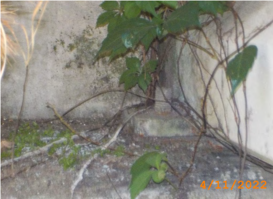
Photo 7: Element 313: South nut missing from Bearing 1-4 at Abutment 1.
