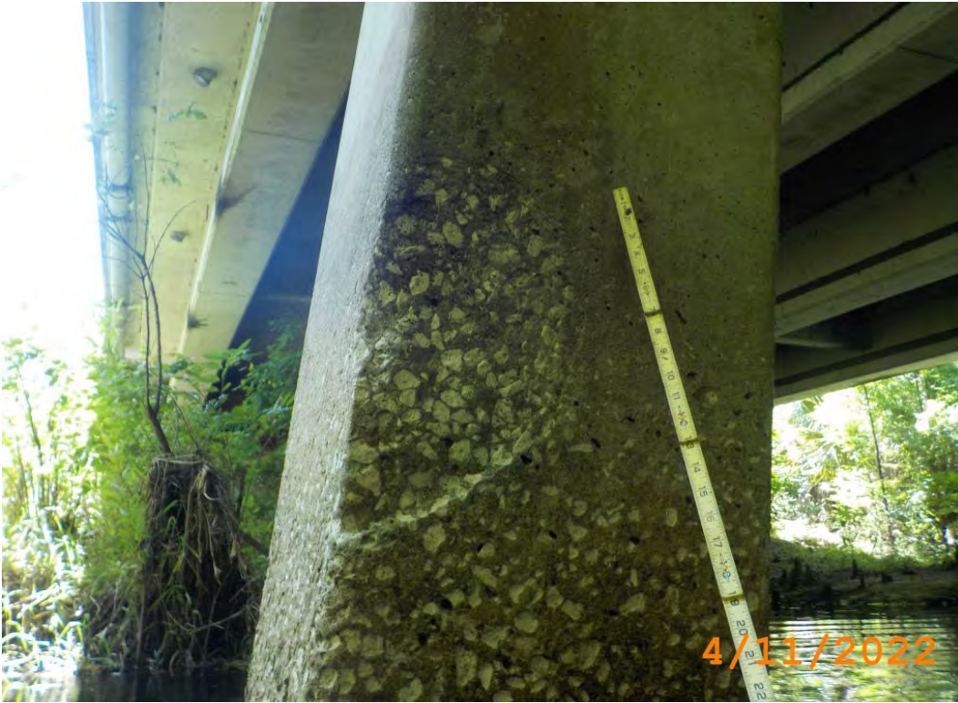
Photo 5: Element 226: Pile 2-4 spall on SE corner, 3ft. below the cap.
