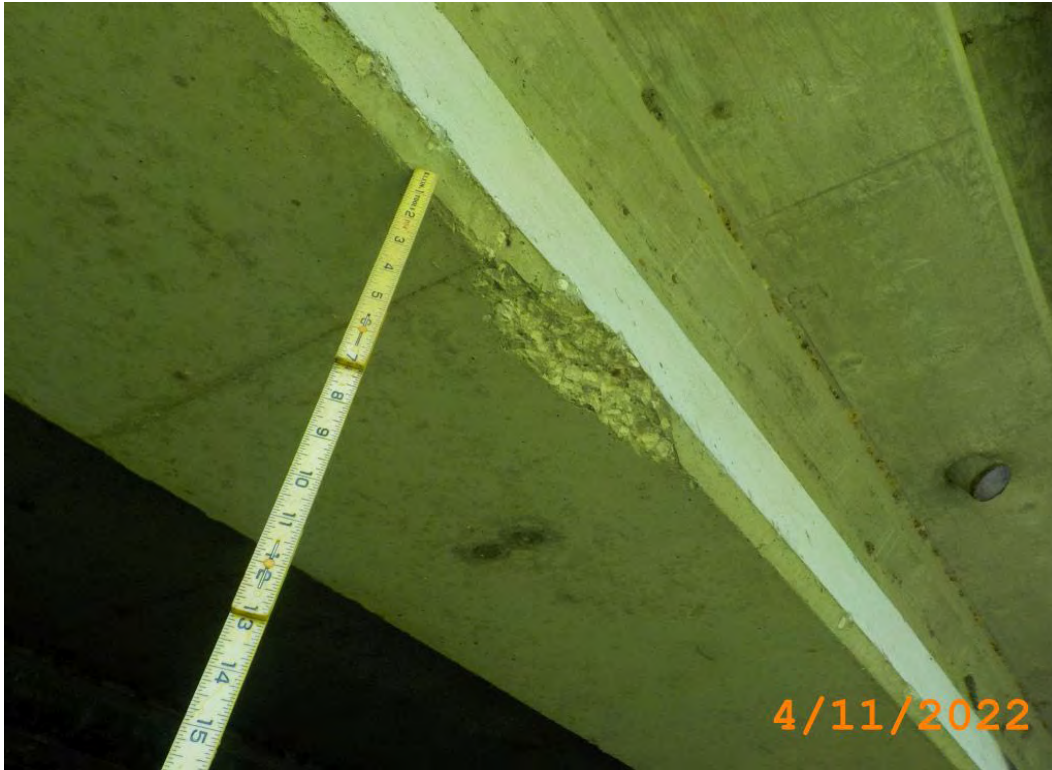
Photo 9: Element 109: Beam 1-4 spall on bottom south edge of flange.
