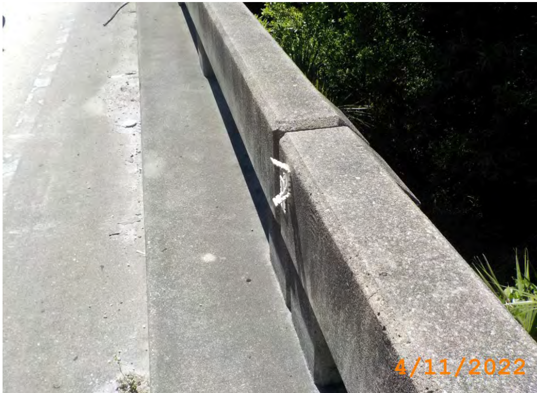
Photo 10: Inspection Notes: Broken bridge rail reflectors.
