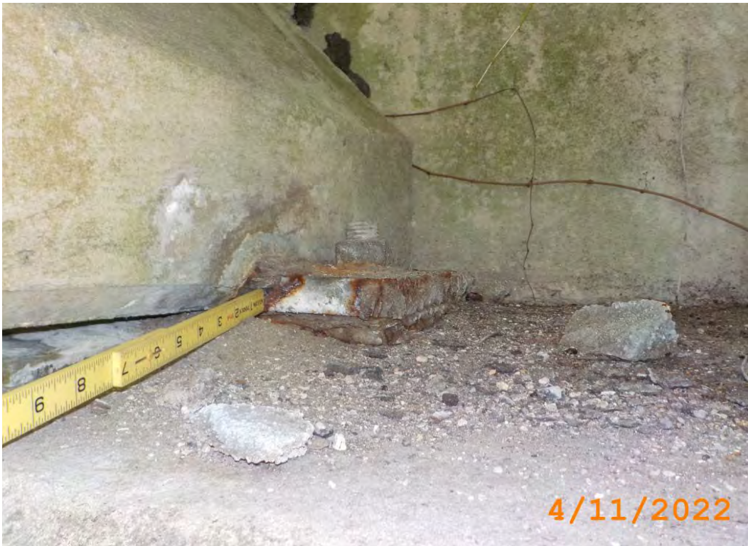
Photo 8: Element 313: Heavy flaking corrosion on Bearing 1-1 at Abutment 1.
