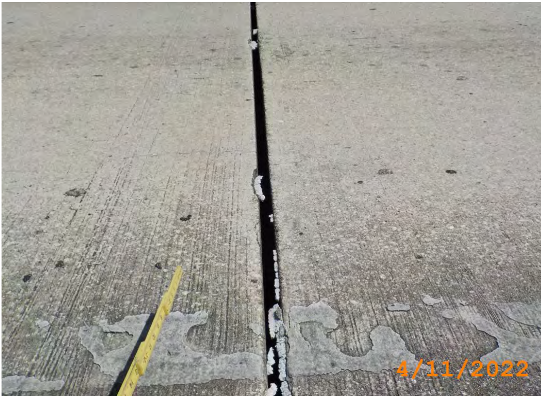
Photo 2: Element 301: Typical failing / missing pourable joint seal.
