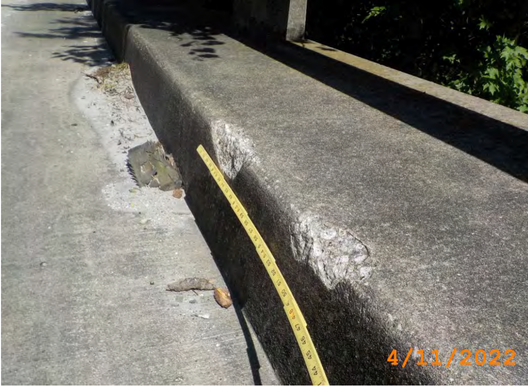
Photo 1: Element 12: Typical impact related spall along south curb.
