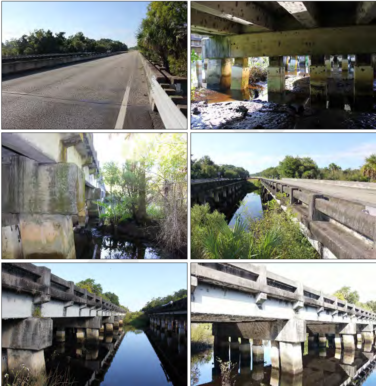
Figure 3. Representative views of Resource 8FL01008/8SJ08262. Deck and roadway, facing southeast (top left); underside with girders and piers, facing southeast (top right); west side of structure, facing south (middle left); railing along east side, facing south (middle right); railing and east side, facing north (bottom left); east side and piers, facing northwest (bottom right).
