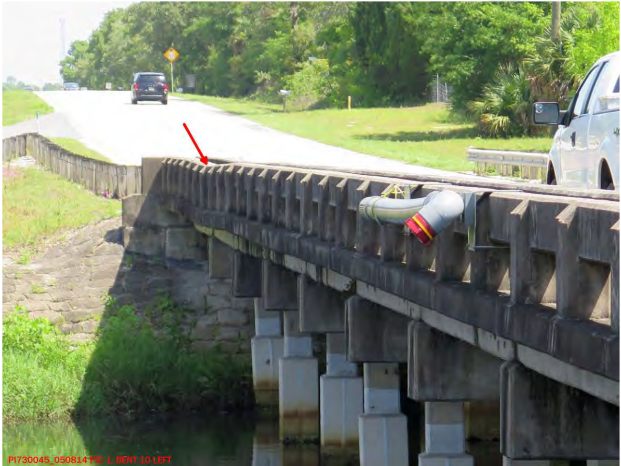
Photo 1: Settlement of bridge no. 730045 – US-1 Northbound over Pellicer Creek
