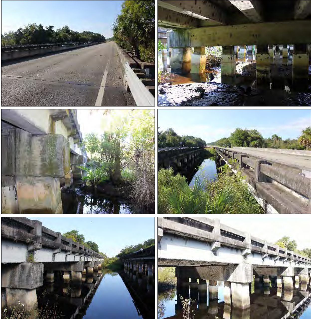
Figure 3. Representative views of Resource 8FL01008/8SJ08262. Deck and roadway, facing southeast (top left); underside with girders and piers, facing southeast (top right); west side of structure, facing south (middle left); railing along east side, facing south (middle right); railing and east side, facing north (bottom left); east side and piers, facing northwest (bottom right).
