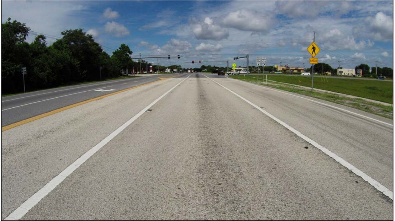
Photo 9: SR 501 northbound near MP 3.295. From MP 3.115 to MP 3.358, the surface course of the northbound R1 lane, outside right turn lane and outside paved shoulder has an open-graded friction course (OGFC) of FC-2 instead of the dense-graded friction found elsewhere on the project.
