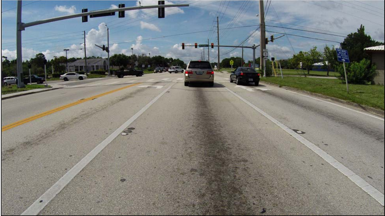
Photo 1: SR 501 southbound near MP 2.283. The pavement surface at the beginning of the project is an older friction course. It is in fair condition with minor cracking distress.
