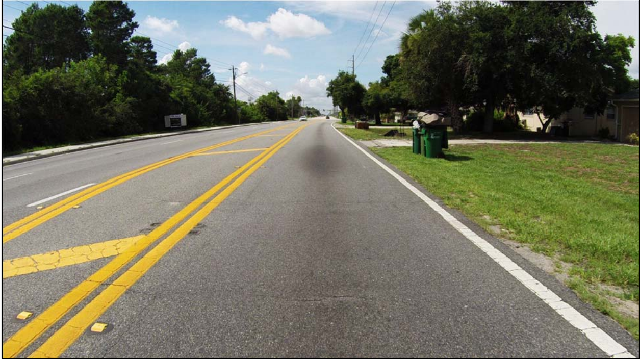
Photo 3: SR 501 southbound near MP 2.468. The center turn lane and southbound L1 travel lane is the original alignment with Sand Bituminous Roadway Mix (SBRM) as a base instead of Limerock.
