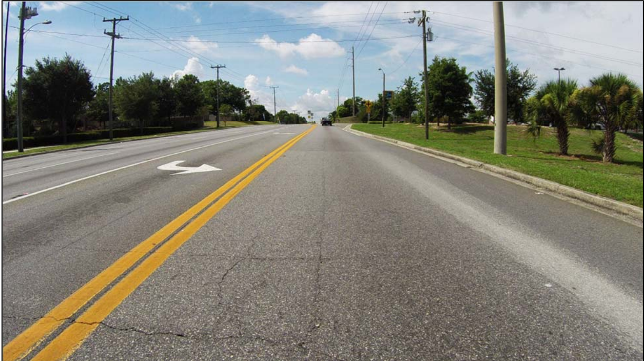
Photo 4: SR 501 southbound near MP 2.650. This is an example of the reflective cracking from the SBRM base of the original roadway base coming to the surface. The outside portion of the lane is widening and has a Limerock base.
