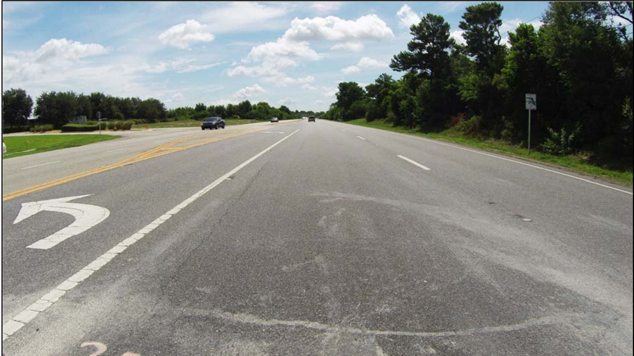
Photo 8: SR 501 southbound near MP 3.263. There are continuous minor longitudinal cracks where pavement joints exist from the last asphalt work on the roadway in 2005.
