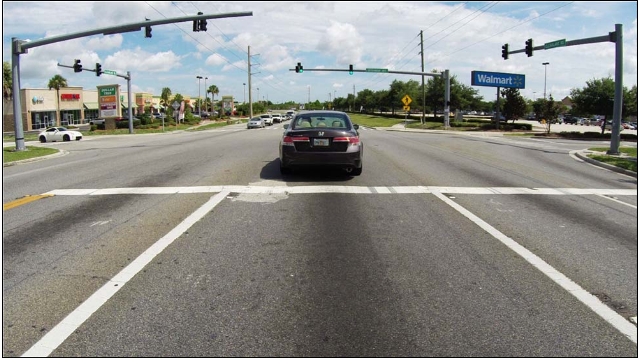
Photo 5: SR 501 northbound near MP 2.655. This is an area of visible rutting in the roadway. Note the asphalt patch at the stop bar. This is at the intersection of Otterbein Avenue.
