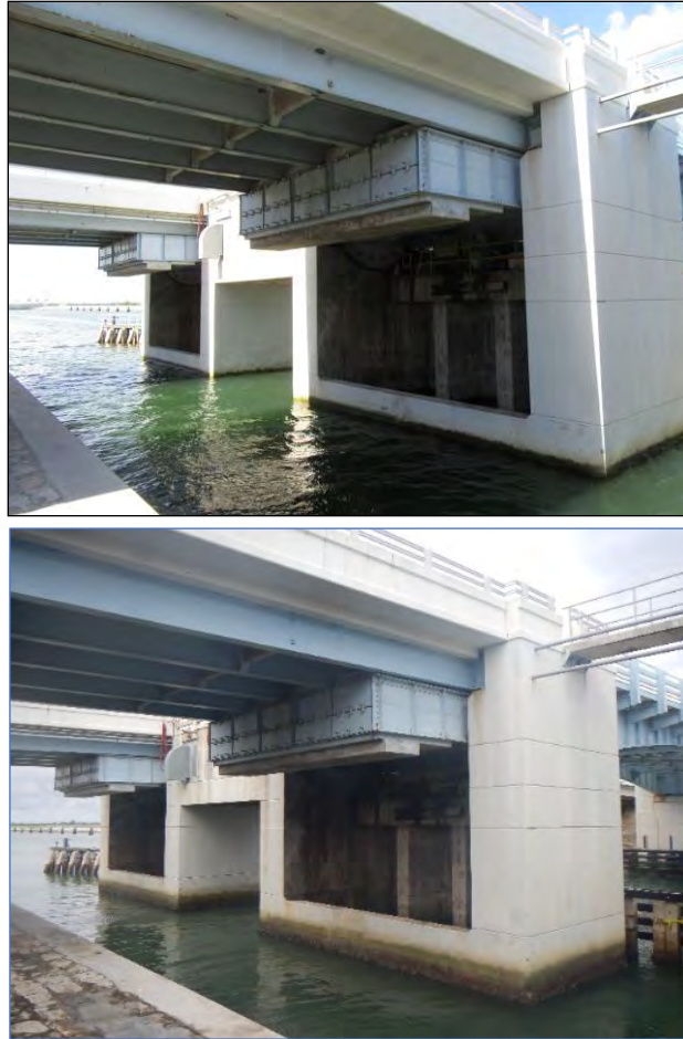
Figure 14. Resources 8BR03009 and 8BR03010 in 2017, facing northwest (top) and in 2021, facing northwest, (bottom).
