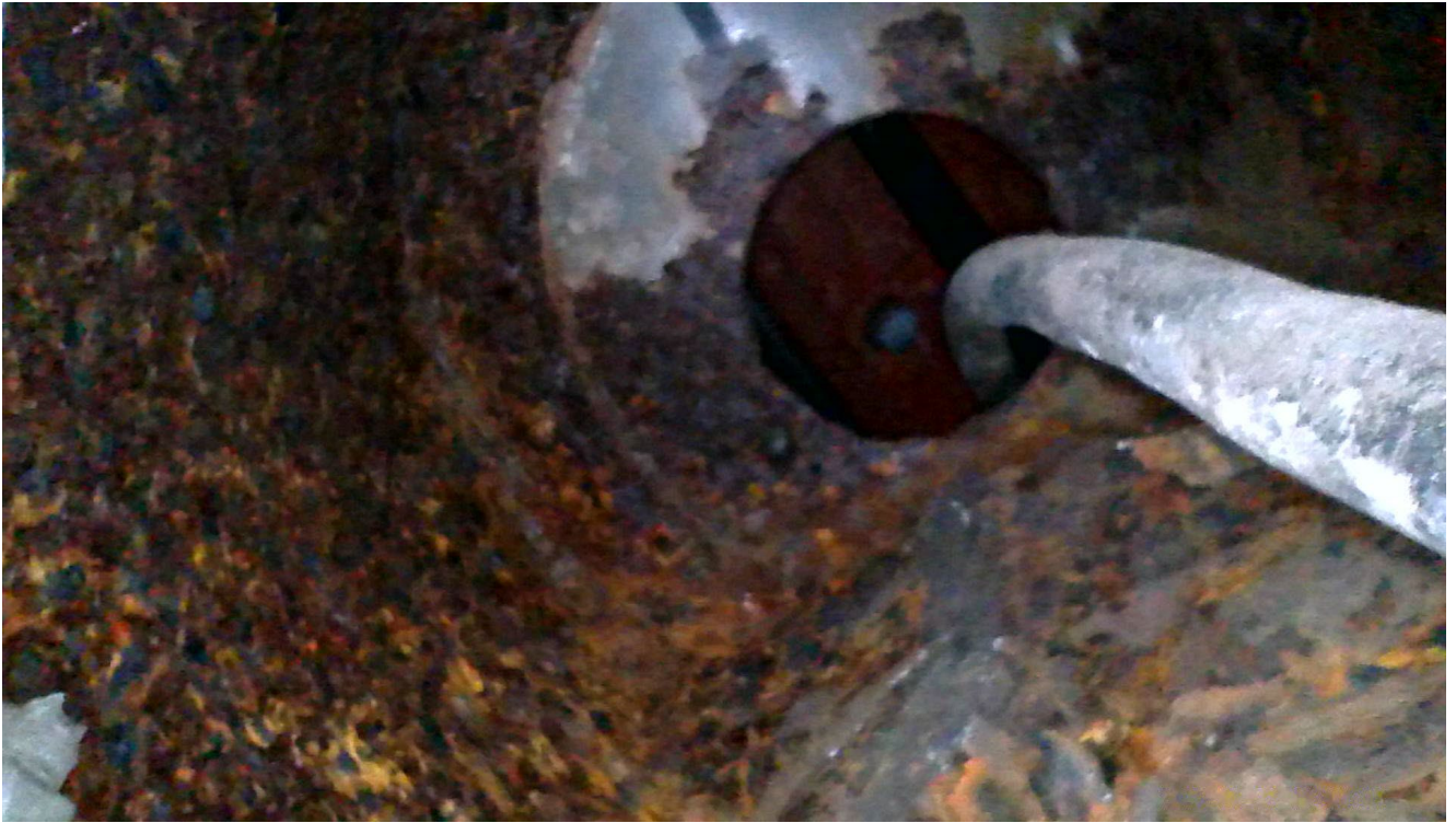
Photo 9: V1/H1 – Borescope view of corrosion on arm interior
