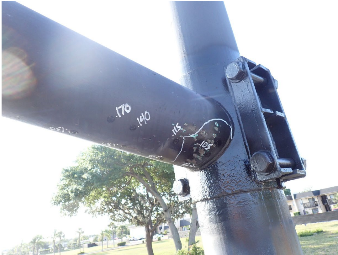
Photo 5: V2/H2 – Thickness readings on underside and west face of arm
