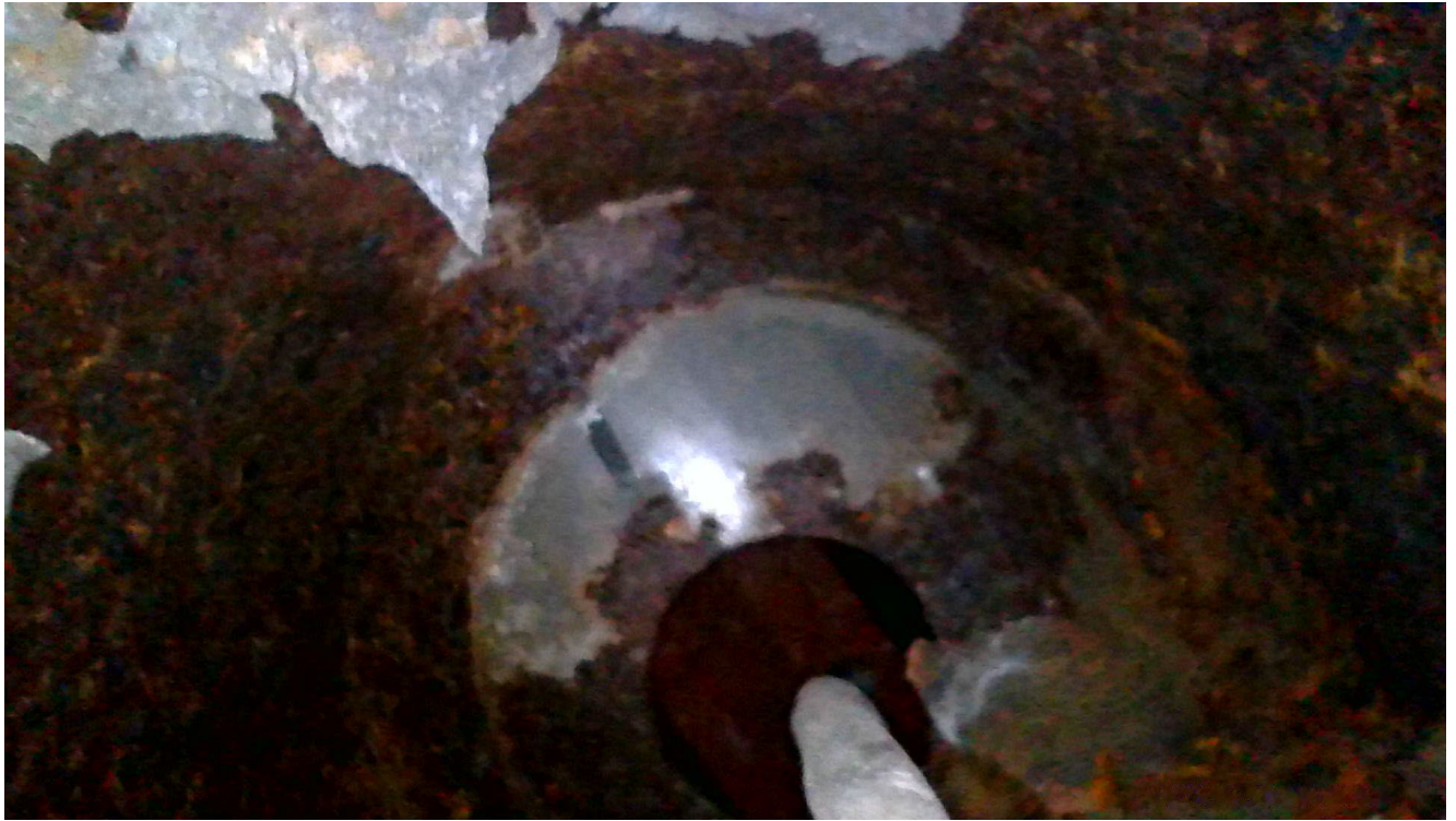
Photo 11: V1/H1 – Borescope view of corrosion on arm interior
