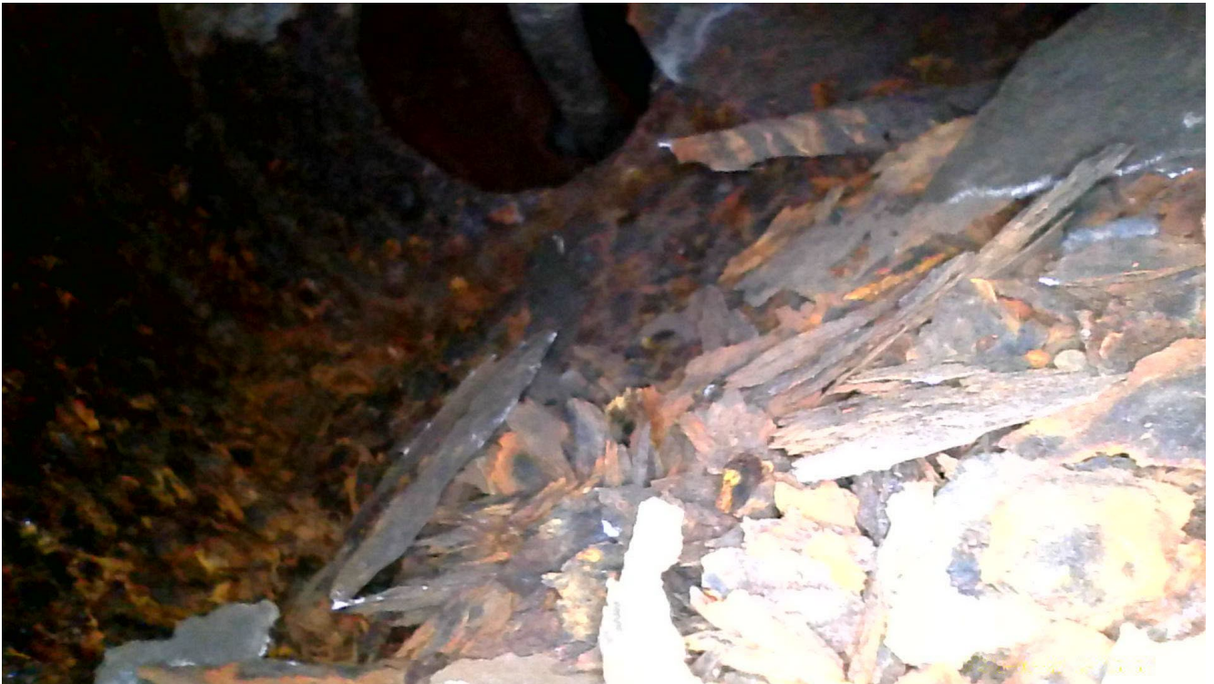
Photo 10: V1/H1 – Borescope view of corrosion on arm interior
