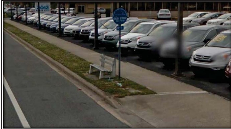
Figure 27: Bus Stop Location Lacking a Paved Landing Pad
